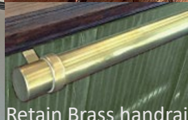
Retain Brass handrail
